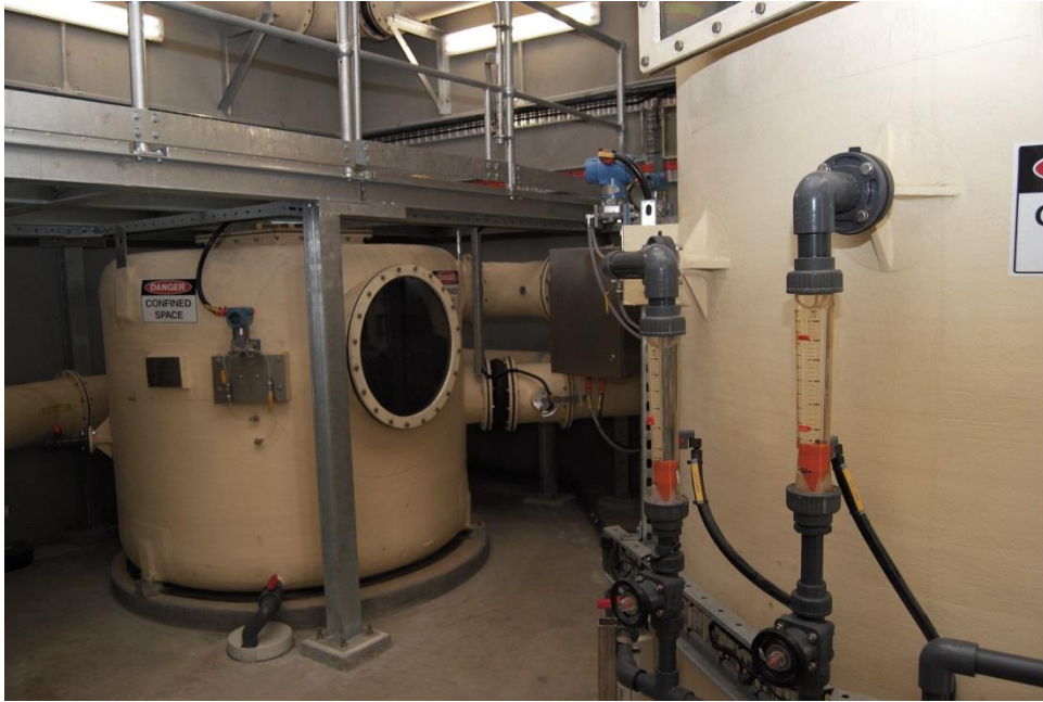
Figure 3: Activated Carbon Filter (one of two units installed)
